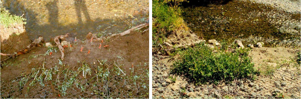
Brush mattresses can be built along the edges of gabion mattresses and can actually be tied into the mattress for better security.
